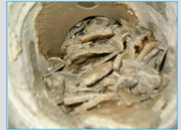
Normal scaling of Lime Kiln Scrubber over a 90 day period
